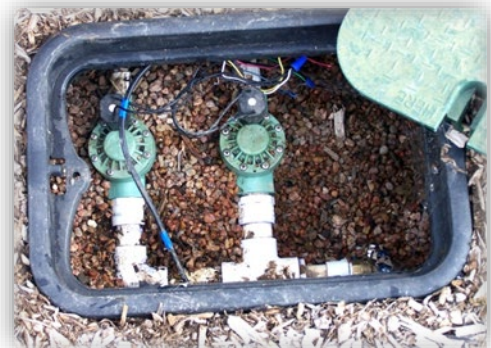
Figure 3. Valve box with two zone valves.
