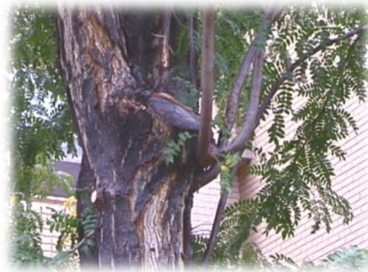
Figure 11. This adventitious sucker growth from a reduction cut is structurally unsound and prone to storm damage as it grows.
