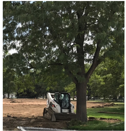
Heavy equipment traffic compacts soils
